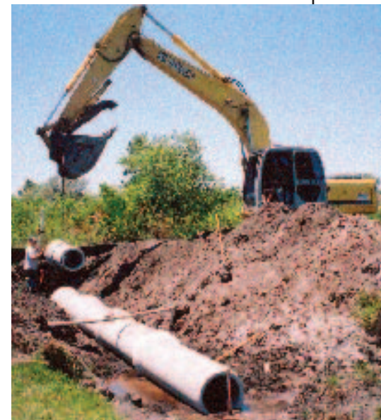
▲ Mizell Landclearing team setting culvert pipes under one of the new roads.
