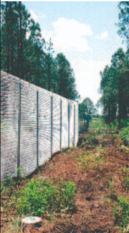
A stretch of fence erected on the south side of the new enclosure. ▼
