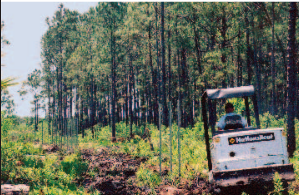
▲ Arrow Fence workers encountered tremendous difficulties installing the posts for the 12' fence surrounding the new 12-acre forest.
